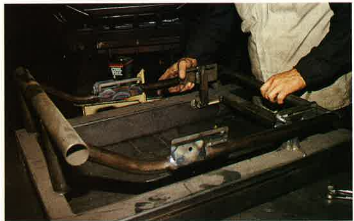
Above: The jigs are used in the placement of the roll cage on the chassis fixture. Notice that interior metal installation has started. Left: This fixture is for seat rails and seat belt brackets, later placed as a complete component in the car and welded. Left below: This lower A-arm fixture incorporates many machined parts, which, like a jig-saw, are cut and fitted to be welded as an assembly.
